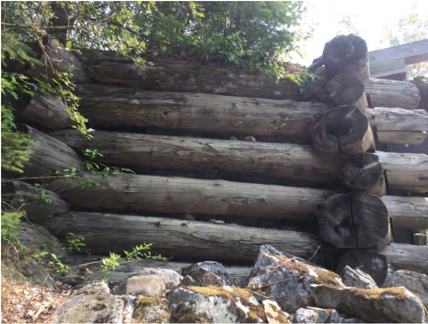
Upstream left approach crib condition
